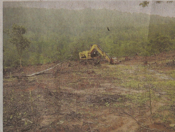
Forestland being levelled using an earth mover to raise a monocrop plantation at Pothumoola under the Begur forest division in Wayanad district.
