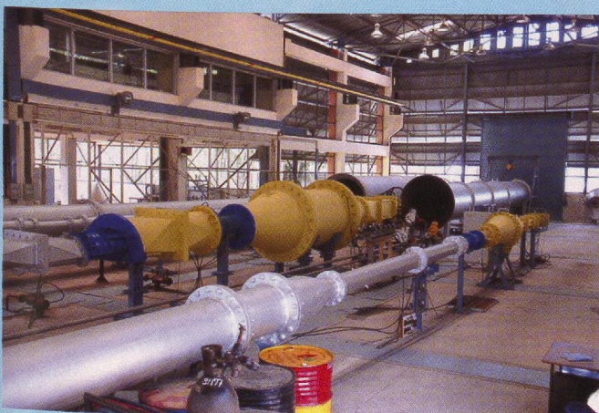
High-Speed Combustor Test Facility.
