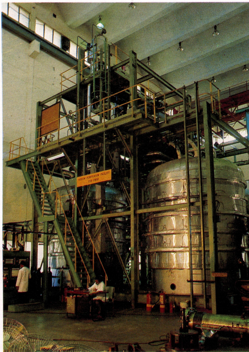
SODIUM PURIFICATION FACILITY
