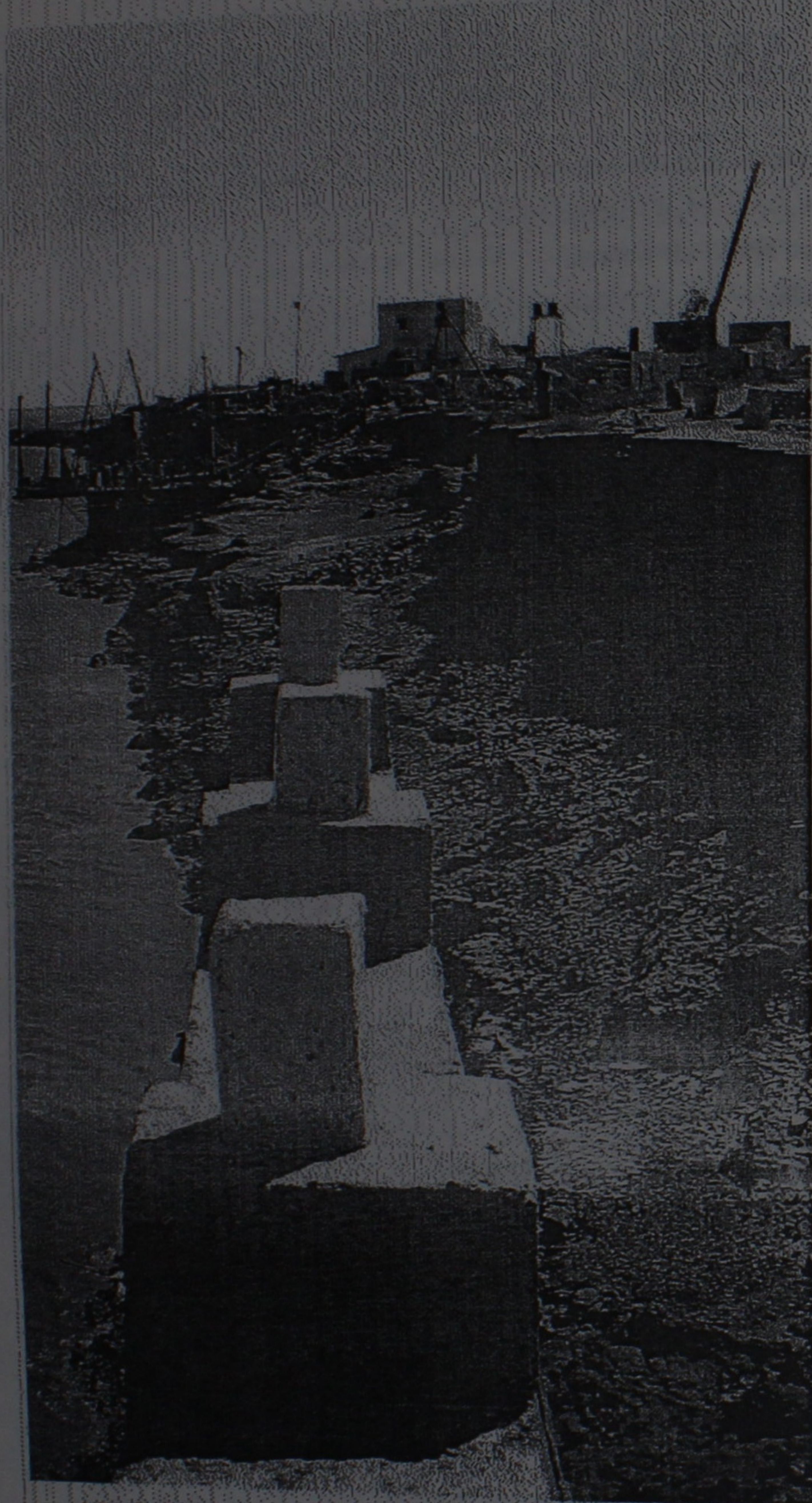
A ROAD BUILT two years ago near Kaladra village has been eroded. A sea wall (in the foreground) offered little protection.
