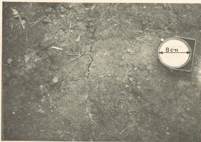
Ground cracks observed near Thalasseri.
